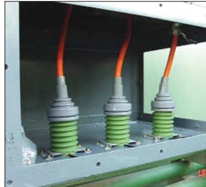
Installed Capacitive Coupler
