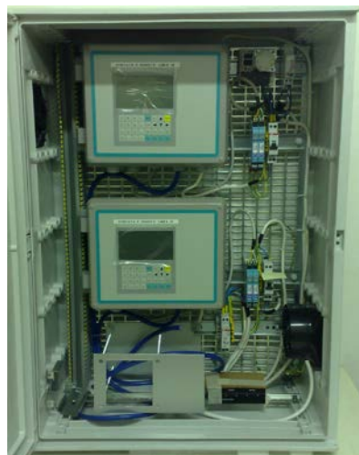
SITE STATION BOX MARE
